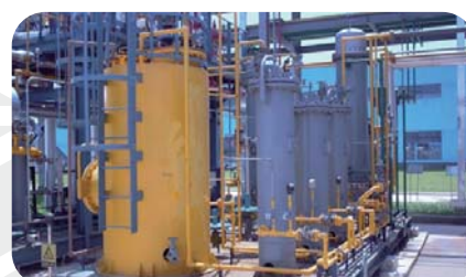
Dehydration and mercury removal Unit
