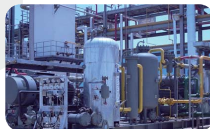
Mixed refrigerant compressor Unit
