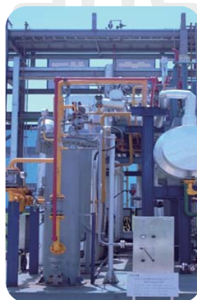
Dust filter Unit
