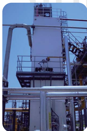
Cold box unit
