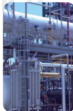
Recycling and reuse of refrigerant Unit
