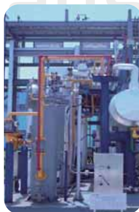
Dust filter Unit
