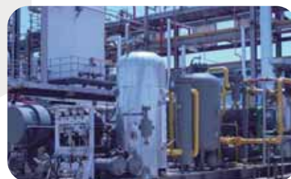
Mixed refrigerant compressor Unit
