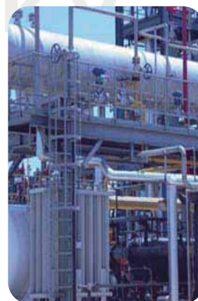
Recycling and reuse of refrigerant Unit
