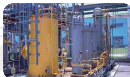
Dehydration and mercury removal Unit
