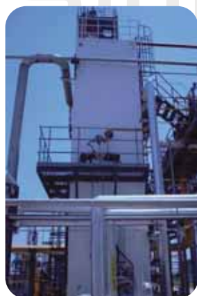
Cold box unit
