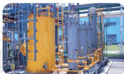
Dehydration and mercury removal Unit
