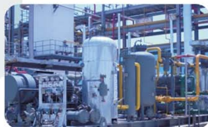
Mixed refrigerant compressor Unit
