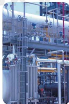
Recycling and reuse of refrigerant Unit
