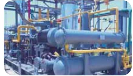
Raw material gas filtration, metering, pressure regulation Unit
