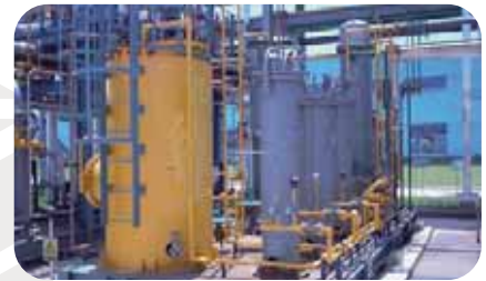
Dehydration and mercury removal Unit
