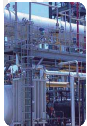
Recycling and reuse of refrigerant Unit
