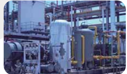
Mixed refrigerant compressor Unit
